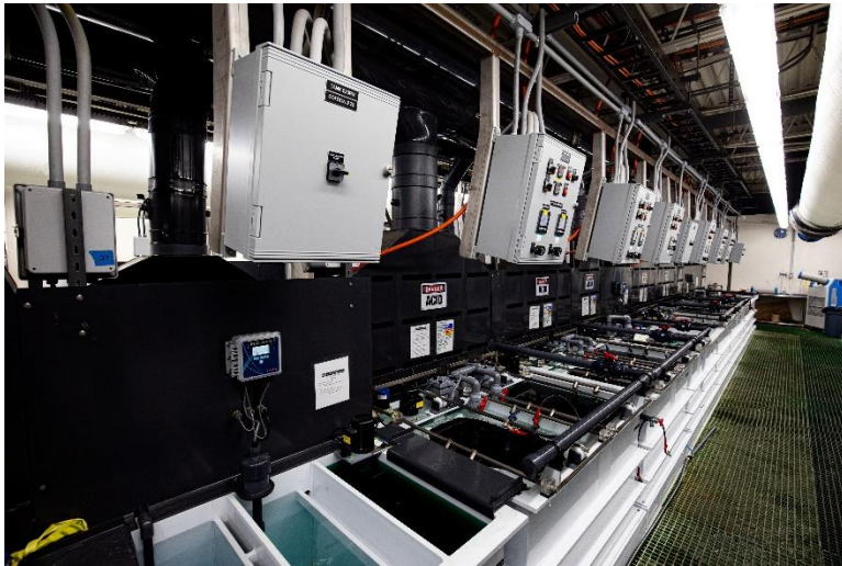
One of the 4 new plating lines in the Cambridge facility Photo Credit: Egide USA
